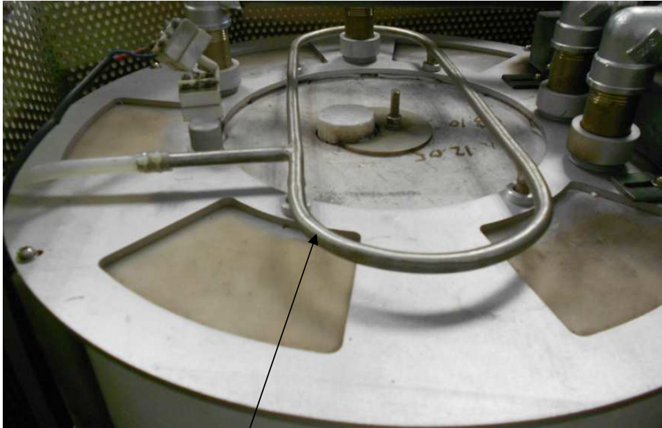
Venting pipe for combustion furnace
